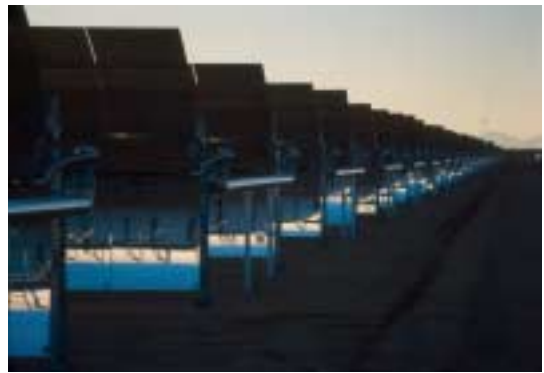
A solar plant in California 1988
